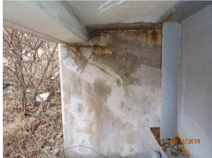
View of minor cracking at the north end of abutment 5's backwall.
