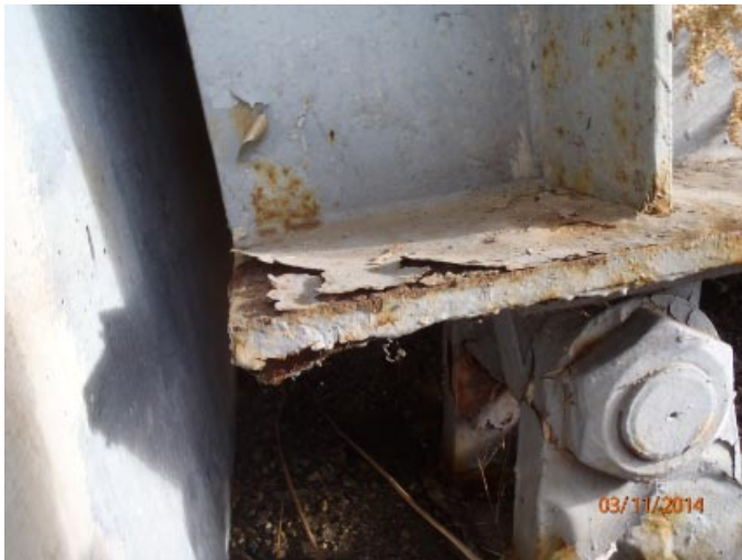
View of flaking paint with minor to moderate corrosion in the bottom flange of the south beam at abutment 1.
