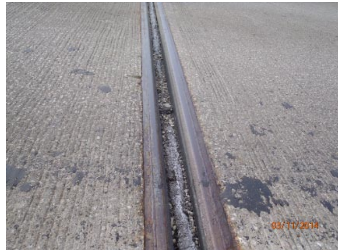
View of the transverse joint over pier 4. It is partially full of debris.
