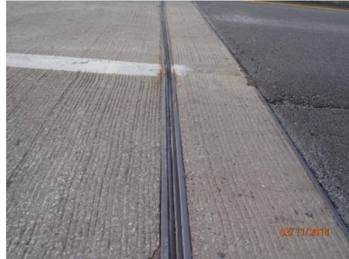
View of the transverse joint at abutment 1. It has some small tears and local adhesion failure.
