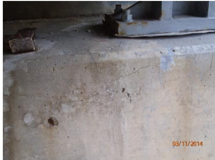
View of minor cracking at the south end of abutment 5's breastwall.
