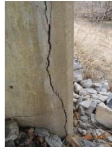
View of moderate vertical cracking (3/8" wide near the ground) in the north face of the south column of pier 4.
