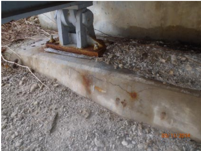
View of minor cracking at the north end of abutment 5's breastwall.
