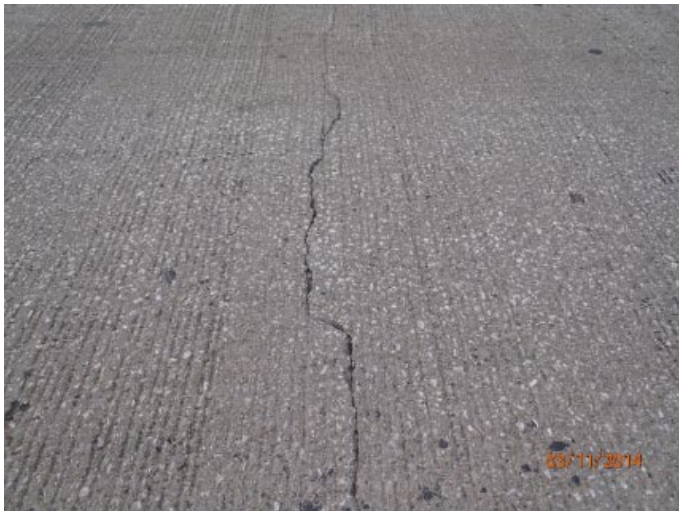
View of some minor transverse cracking in the wearing surface in span 1.
