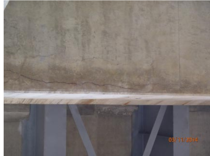
View of minor cracking in the underside of pier cap 4.
