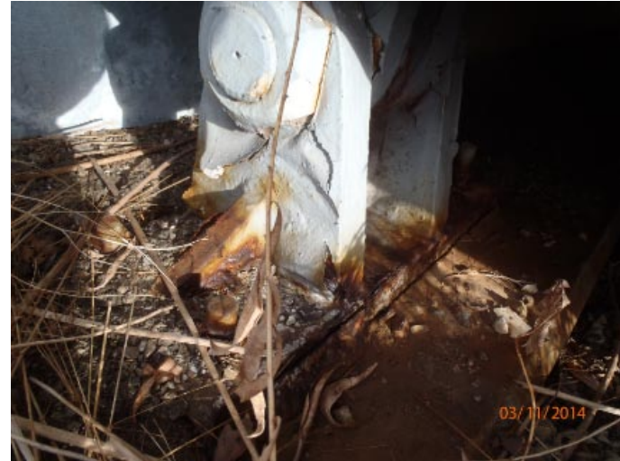
View of the south bearing at abutment 1. Moderate to heavy corrosion is present in the masonry plate and anchor bolts.
