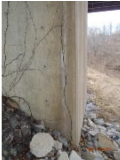
View of moderate vertical cracking (3/8" wide near the ground) in the north face of the south column of pier 4.
