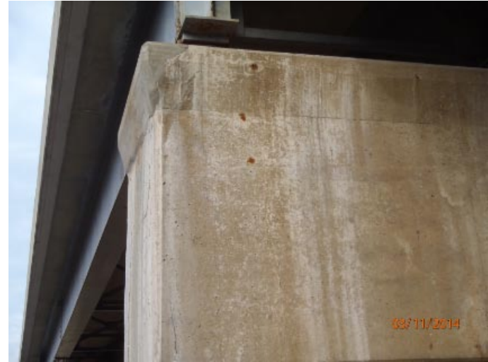
View of minor to moderate cracking at the south end of pier cap 4 in span 4.
