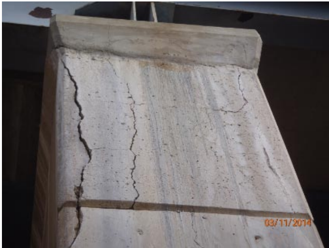
View of moderate to heavy cracking at the south end of pier cap 4.
