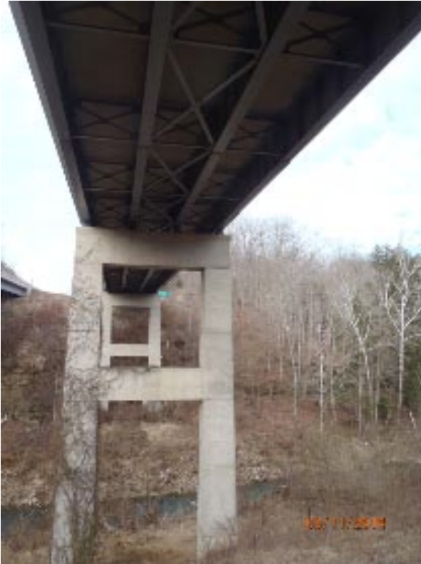
View of span 3 and pier 3. Notice the vines growing on the south column.
