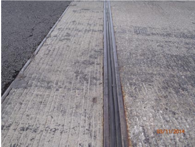
View of the transverse joint over abutment 5. It has some local adhesion failures.
