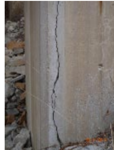
View of moderate vertical cracking (up to 3/16" wide near ground) in the south face of the south column of pier 4.
