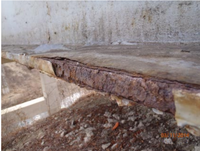
View of flaking paint with moderate corrosion along the bottom flange of the north beam in span 1.
