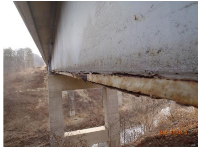
View of flaking paint with moderate corrosion along the bottom flange of the north beam in span 1.
