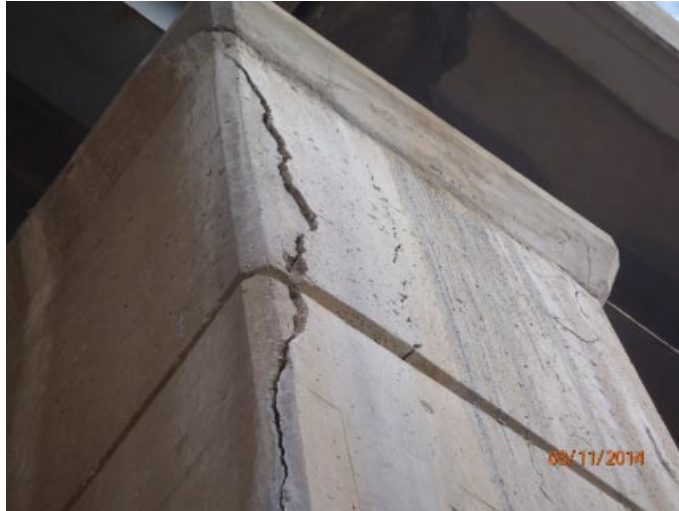
View of moderate to heavy vertical cracking (up to 3/16" wide near ground) in the south face of the south column and cap of pier 4.
