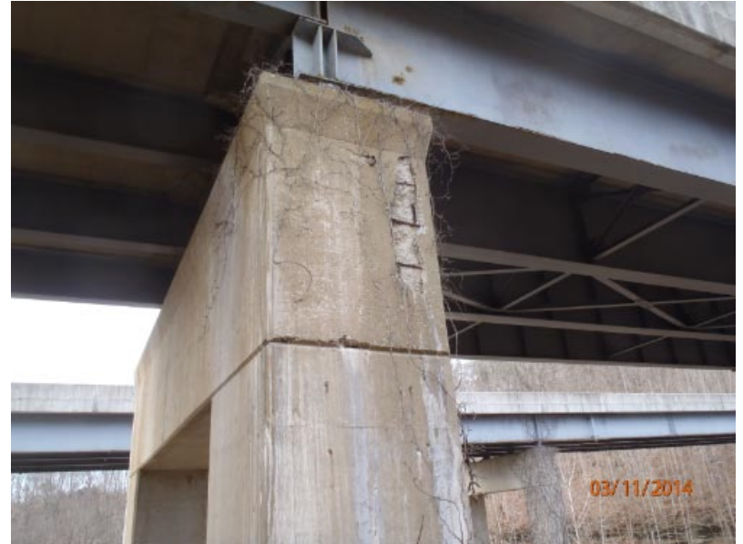
View of a moderately sized and moderately deep spall with exposed steel at the north end of pier cap 4.
